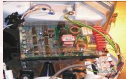
The Active Reactor in Sylvania Roadster 250W HPS Fitting, installed in Springvale Rd
