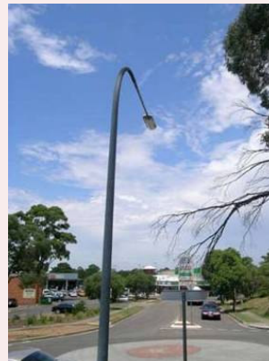
T5 installation as part of NAGA/AGL trials
